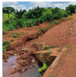
Photos 48: Absence de drainage
