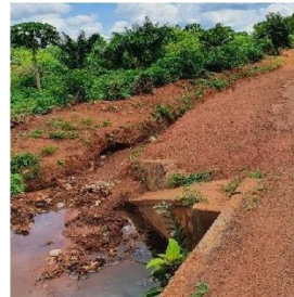
Photos 48: Absence de drainage
